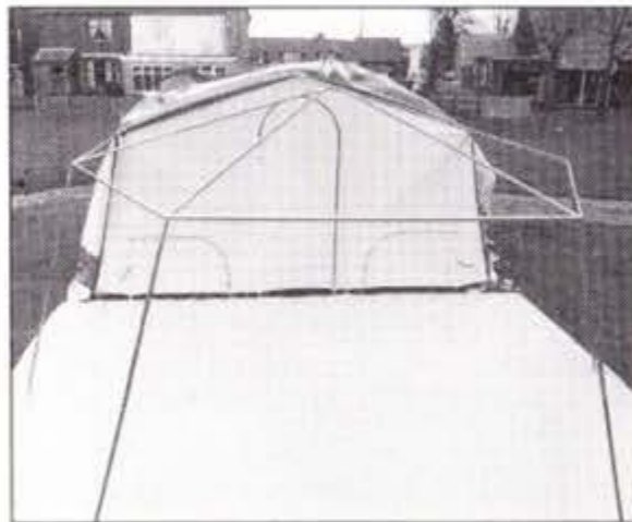
7. Connect the front frame to the four angled roof poles. Level the height of the frame by using the adjustable feet.
